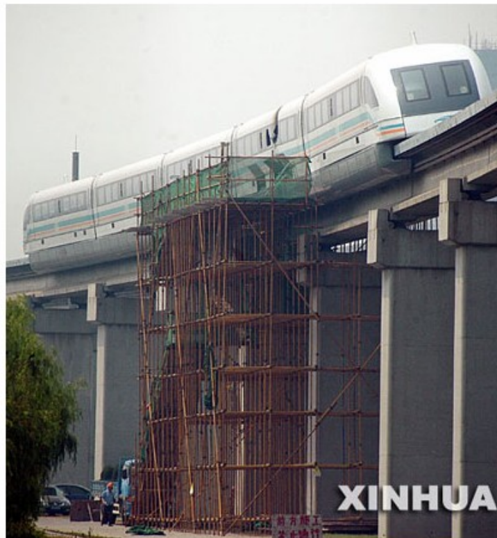
Scaffold is set up close to a magnetic levitation (MagLev) station for MagLev train repair in Shanghai of east China, Aug. 14, 2006. The train was damaged during a fire on the afternoon of Aug. 11.
