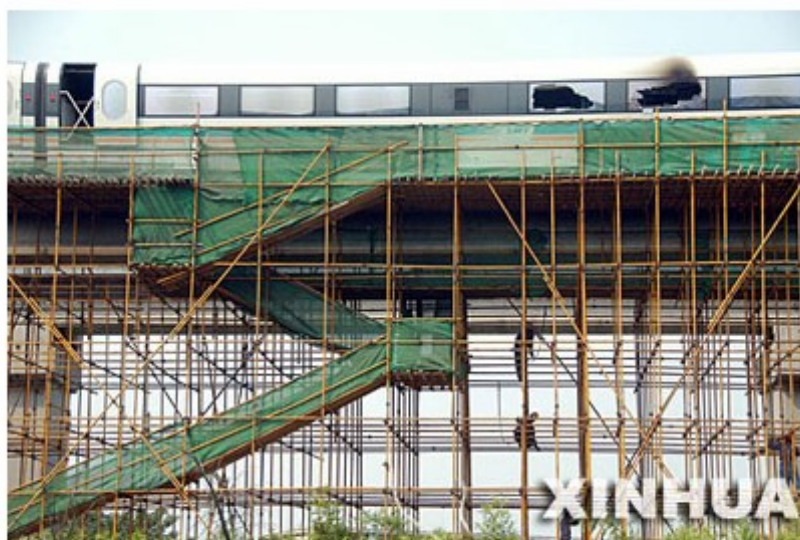
Builders set up scaffold near a magnetic levitation (MagLev) station to repair a MagLev train in Shanghai of east China, Aug. 14, 2006. The train was damaged during a fire on the afternoon of Aug. 11.
